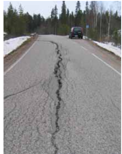
Figure 2. Longitudinal crack caused by differential frost heave in road 19773 in Rovaniemi, Finland.
