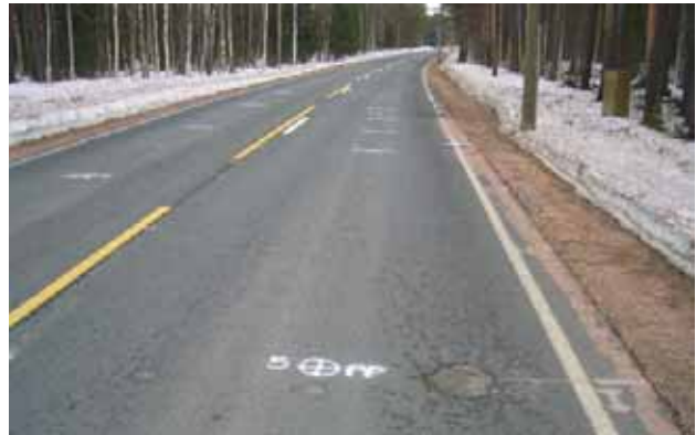
Figure 30. Koskenkylä Percostation site near Rovaniemi. The right lane (in this photo, left lane in survey) lead towards Rovaniemi. FWD points are marked with white paint.
