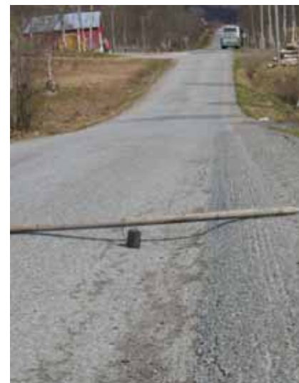
Figure 3. Permanent deformation in road 229 in Senja Norway.
