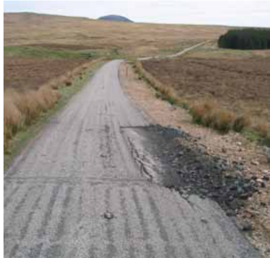
Figure 45. Pavement failures at B871 in early May 2003.
