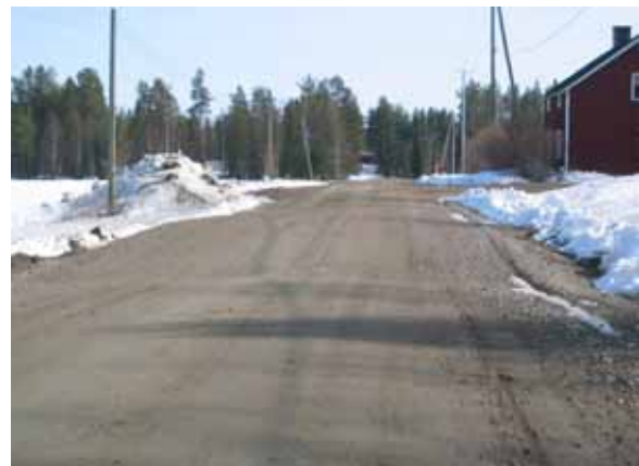
Figure 31. Uneven frost heave bump around a culvert on road 19783 in Kemijärvi. The average frost heave on both sides of the culvert, which has a good foundation and is not heaving, is 40 – 50 cm.
