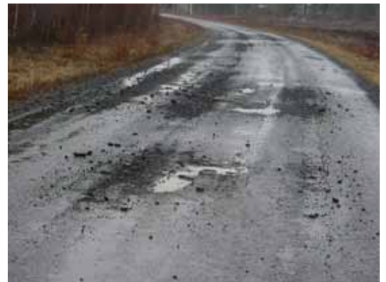
Figure 17. Spring thaw damage on a road with surface dressing in Northern-Karelia in Finland. Photo Martti Leppänen.
