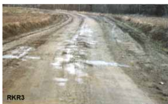
Figure 27. Example of Finnish spring thaw structural damage class 3 on a gravel road. (Painorajoitusohje 2004)
