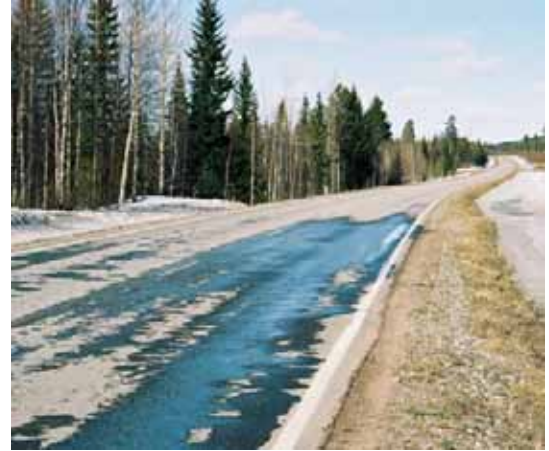
Figure 16. Water breaking through the asphalt from the thawing base course during early spring 2004 in Finnish Lapland.
