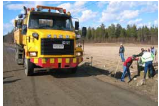
Figure 81. Full scale loading test done at the Kemijärvi Percostation test site using a maintenance vehicle. Behind the truck an area where water is being squeezed to the road surface can be seen.
