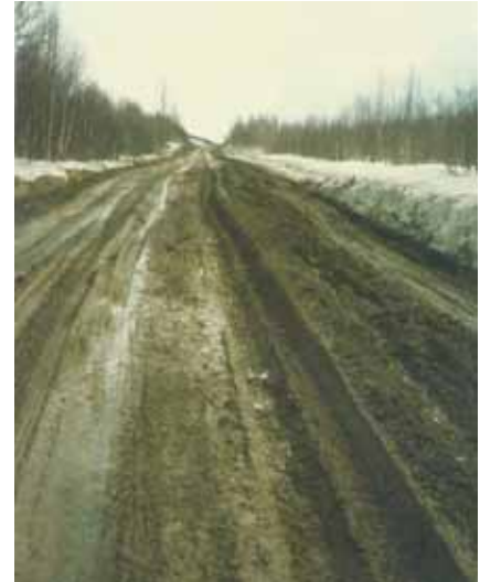
Figure 7. Typical spring thaw damage section on a gravel road near Troms in Norway.
