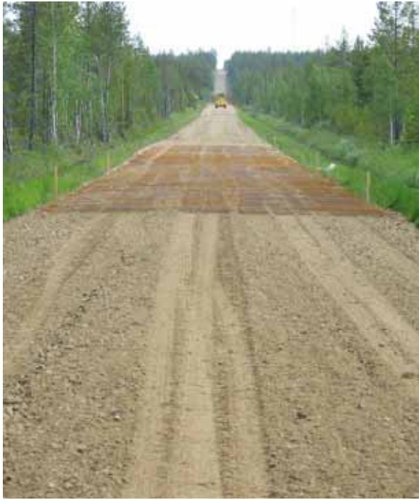
Figure 100. Using steel reinforcement in strengthening a typical spring thaw damaged section on road 955 in Kittilä, Finnish Lapland (photo: K. Niva).
