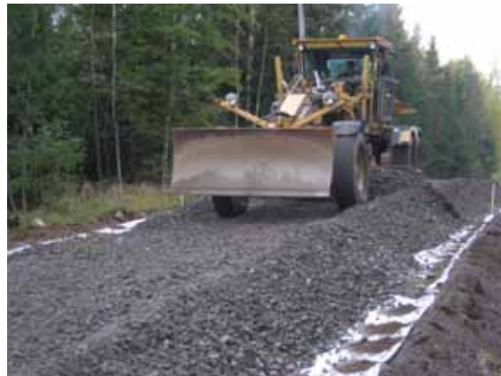
Figure 108. Placing base course over geotextile. Boulders removed during the process of homogenization can be seen on the road shoulder.
