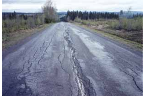
Figure 105. Typical damage on a road that has had spring thaw problems when it was a gravel road (see figure 103) and was paved without homogenization of the old structures and without improving the road structures to an adequate level.
