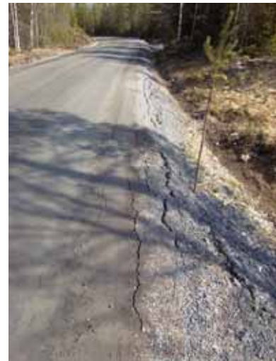
Figure 113. Failure on road shoulder. (photo: P Karhu)
