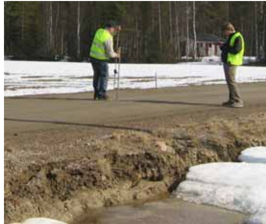
Figure 79. A weak left road shoulder in South side of the road in April 29 th 2003 in Kemijärvi.
