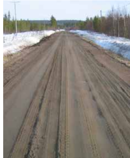
Figure 94. Surface thaw weakening on road 19778 in Kemijärvi Finland. Photo has been taken on 19.04.2004 when the frost had thawed to a level of 120 – 140 mm.
