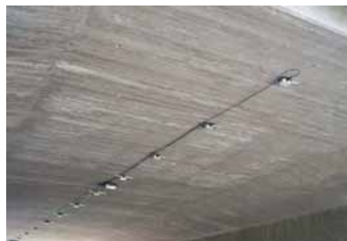
Figure 123. SiWIM sensors instrumented onto the bottom of a bridge. (Photo from VVPubl 2003:5)
