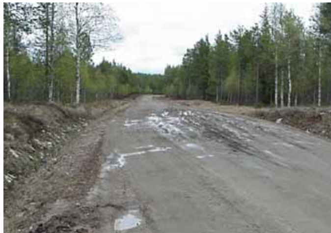
Figure 14. Structural spring thaw damage on road 9613 in Kemijärvi, Finland in 27.5.2003. The subgrade soil is moraine. Notice the widening of the damaged area. Photo:Tarmo Posti.
