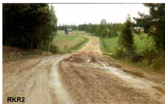
Figure 26. Example of Finnish spring thaw damage class 2 on a gravel road. (Painorajoitusohje 2004)
