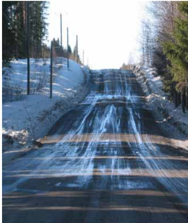
Figure 13. Typical location of surface thaw damage on a hilly area. In the course of basic maintenance graders push wearing course materials from the hilltops to the valley bottoms where wearing course thickness can, over time, increase to 150 – 300 mm. A thick wearing course together with water from the melting snow and vehicles loads causes the road surface to become plastic. (photo: S. Kohonen)
