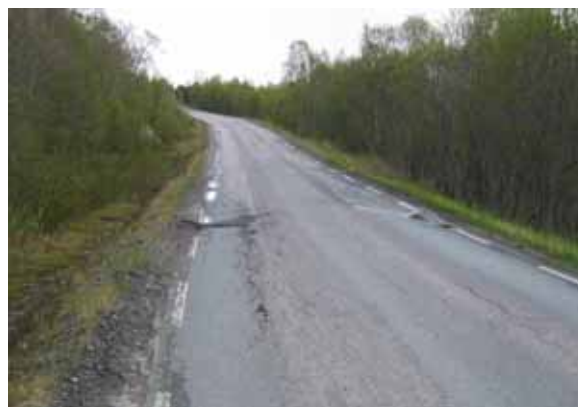
Figure 18. Spring thaw weakening damage on a paved road in Senja, Norway.
