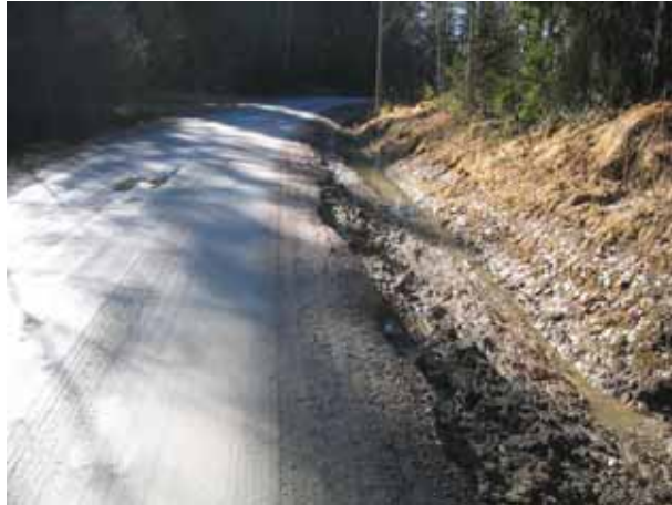
Figure 3.5. The collapsed road shoulder in silty area. The shot was taken during first spring after ditch cleaning.
