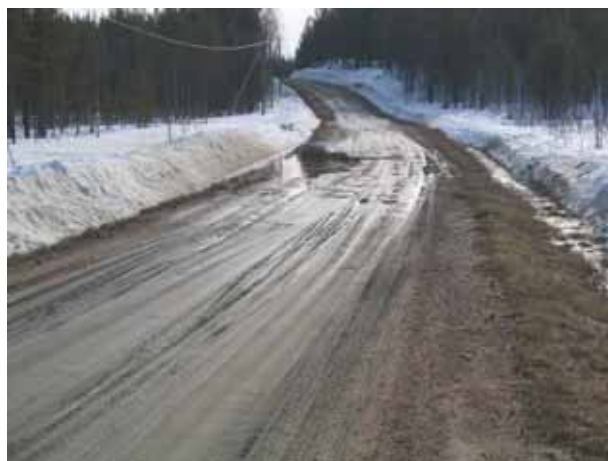
Figure 3.8. Drainage problem on low lying ground, Rd 19778, Kemijärvi, Finland.
