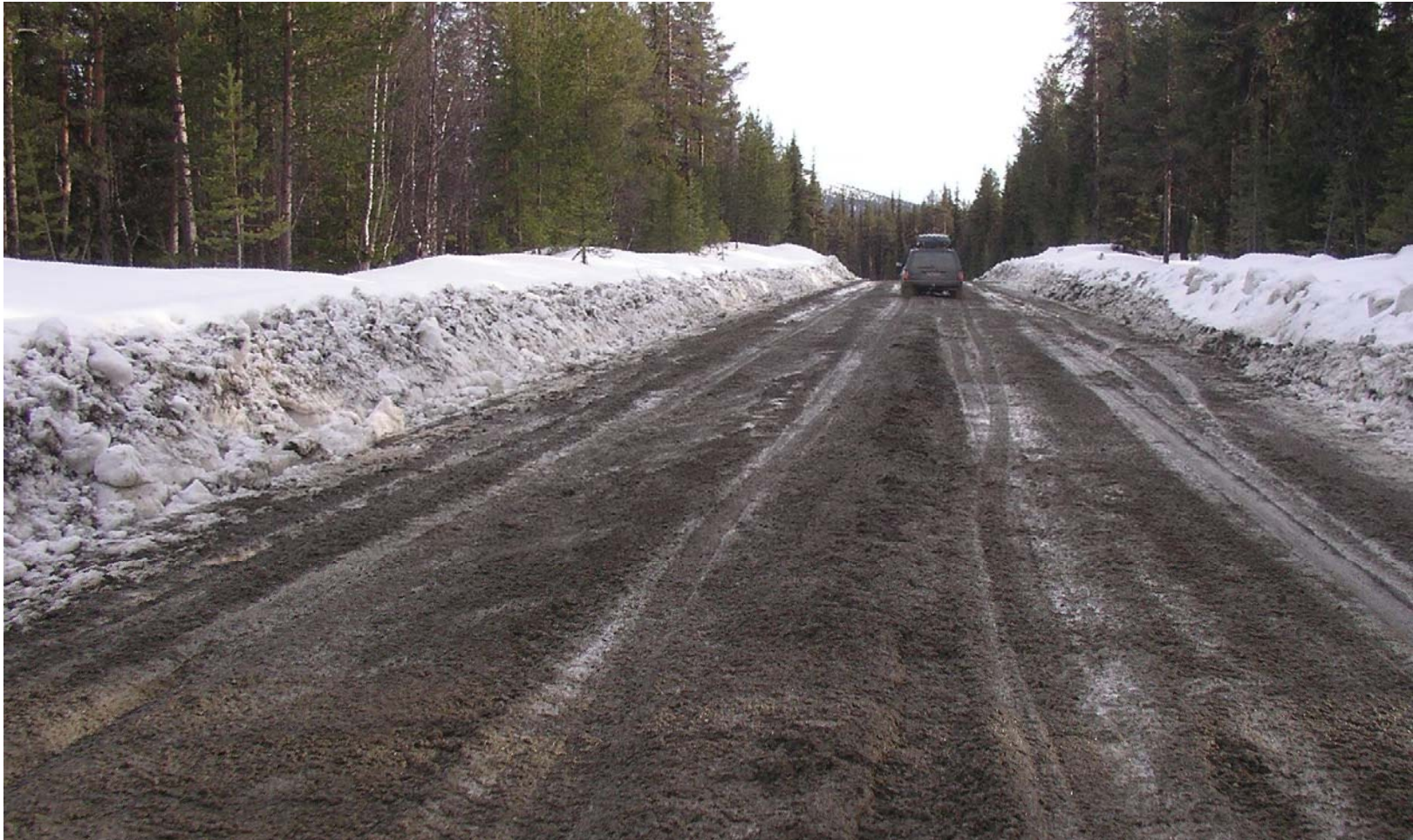
Frost damage on a gravel road in Raattama. Photo J. Leskinen
