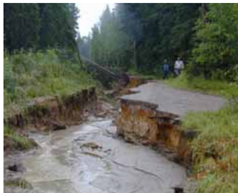
Figure 6. Heavy rains can cause major erosion problems on low volume roads if the drainage system is not working well
