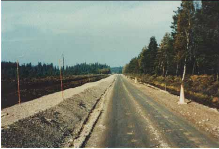
Fig 6.11 Photograph of a widening of a floating road over peat by preloading.
