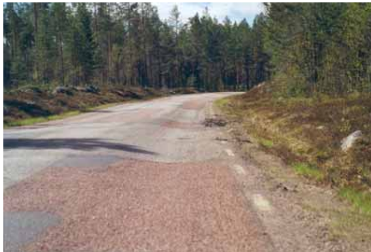
Figure 4.2 Rutting on a small paved road in Northern Sweden.
